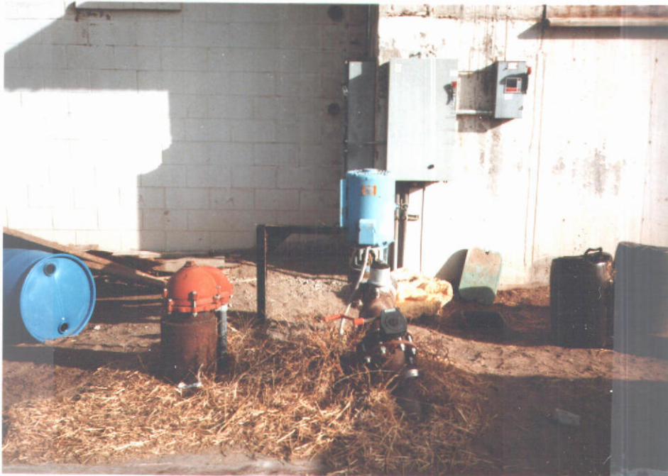
Large Well, Booster Pump
