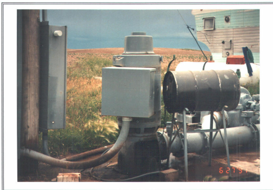
Picture 2 - main pump (200 hp operating at 72 psi)
