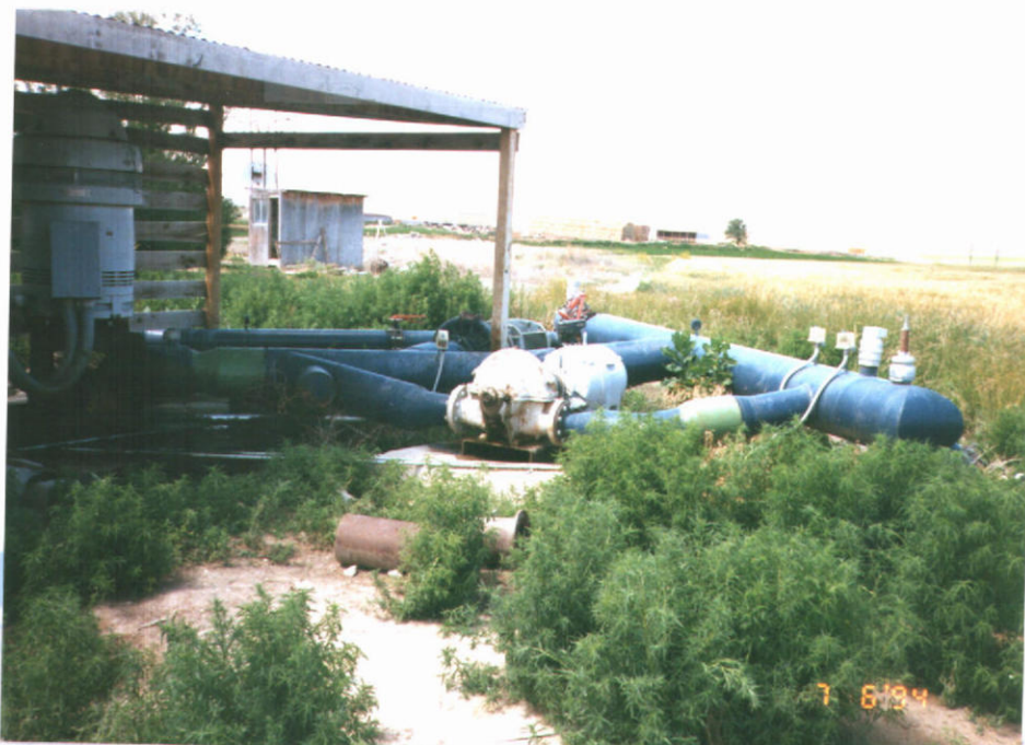
#1 P/O Pump Station #1
