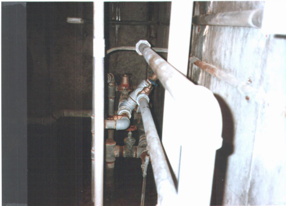
Pipelines From Main Well
