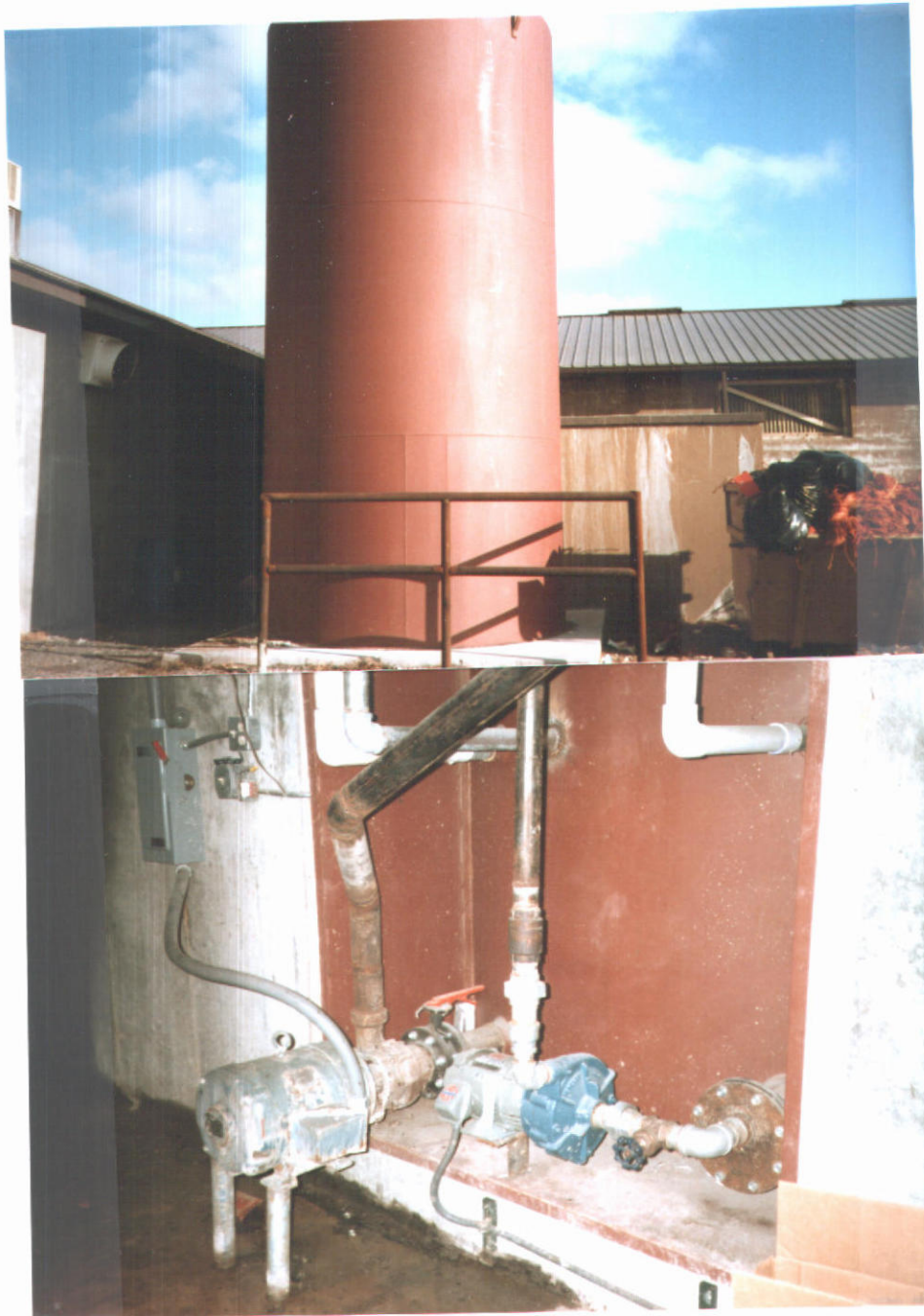
Pressure Pumps From Large Tank
