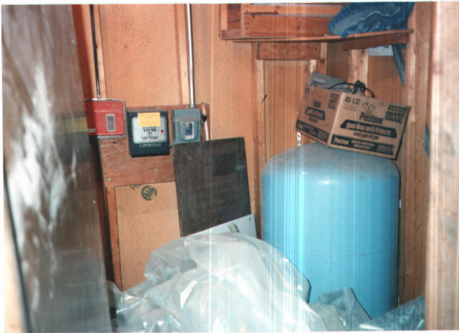
Pressure Tank & Control Box for System -
