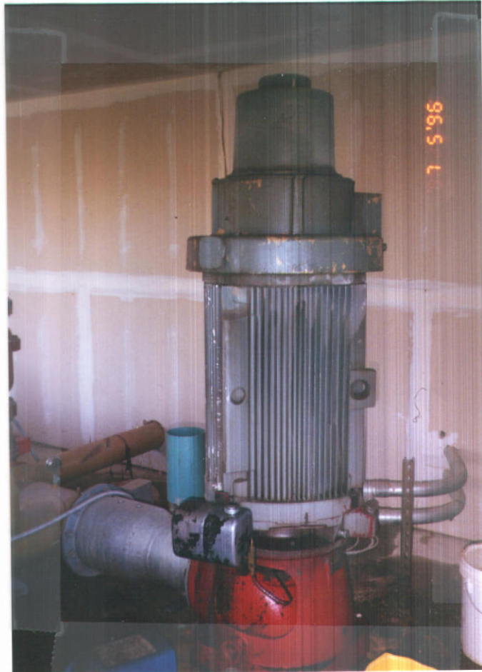
Pump FOR Fire well
