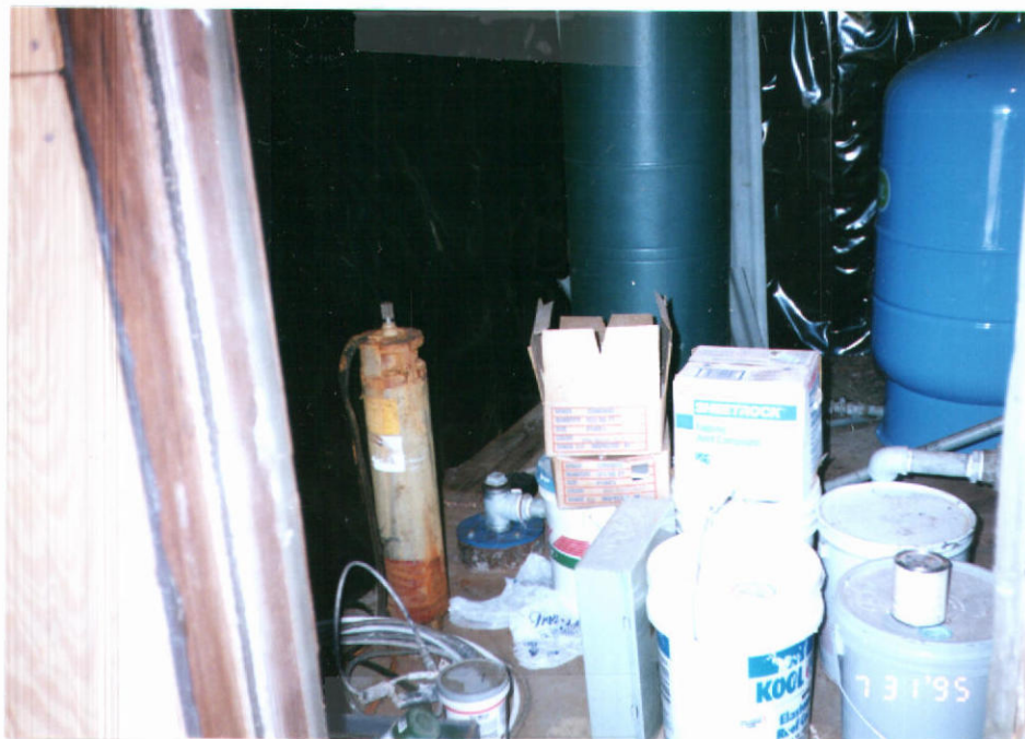
P/D ( Well head & pressure tanks, inside of well house )
