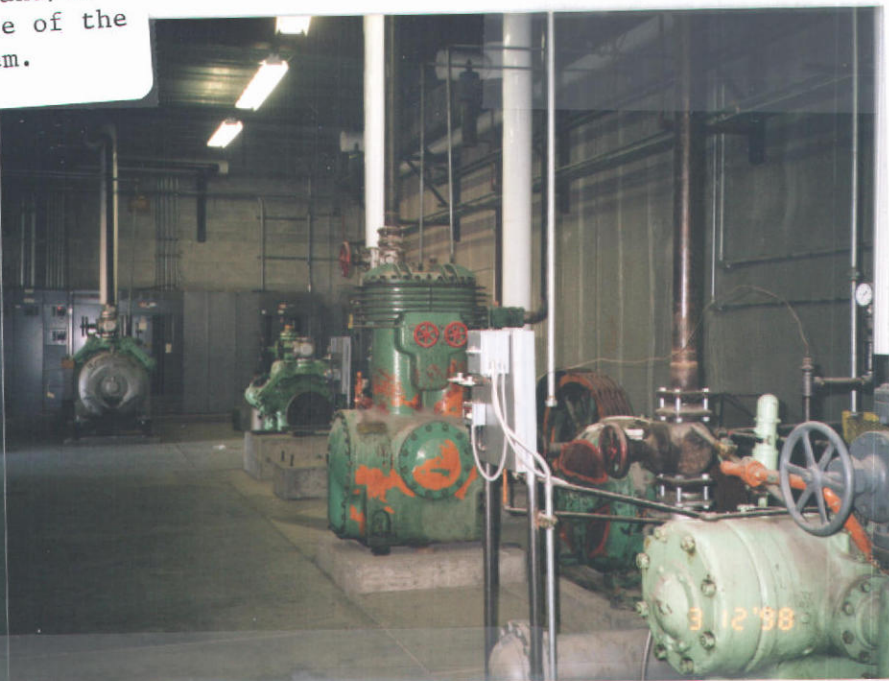
cold storage recovery tank low pressure receiver boiler
