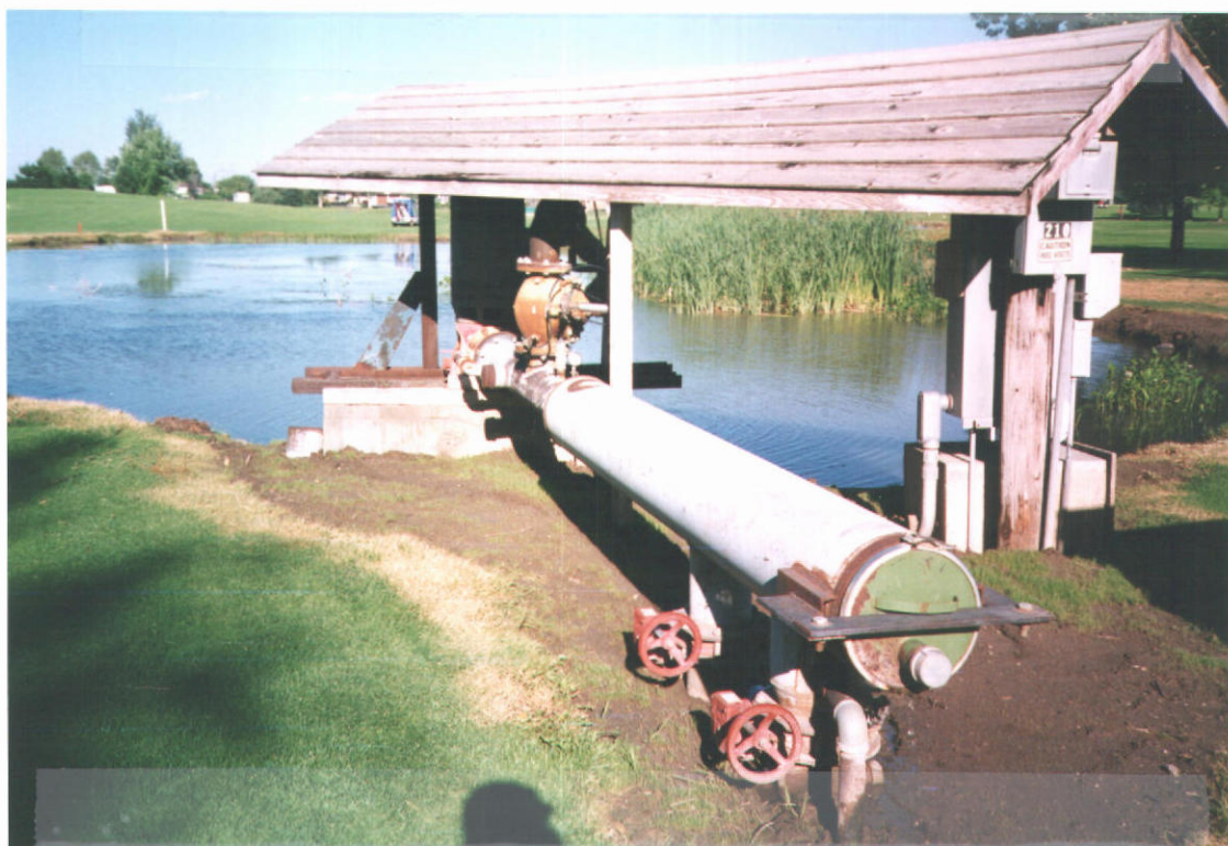
Outlet of West Pump To Buried Sprinklers
