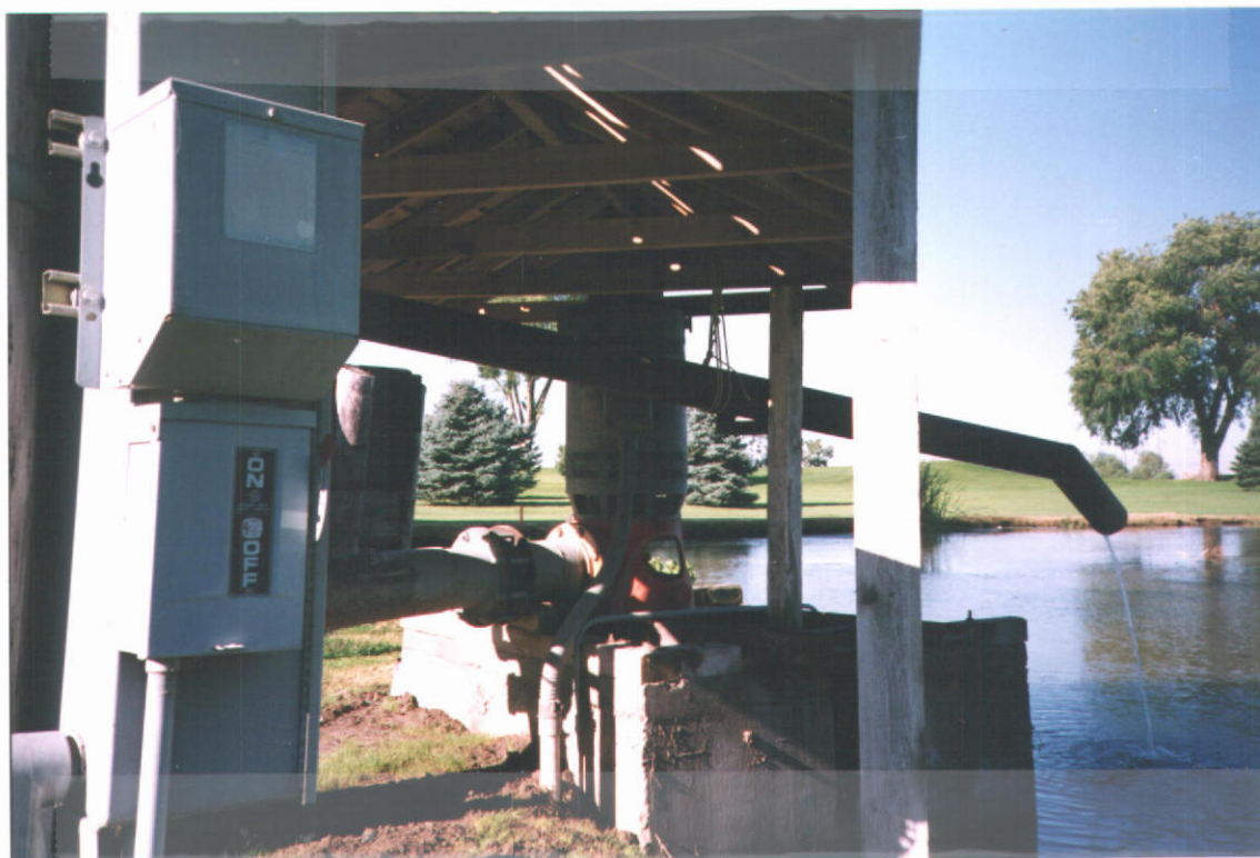
Pressure Pump In West Pond
