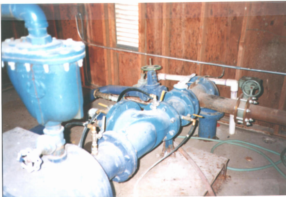
outlets of Re-lift Pumps
