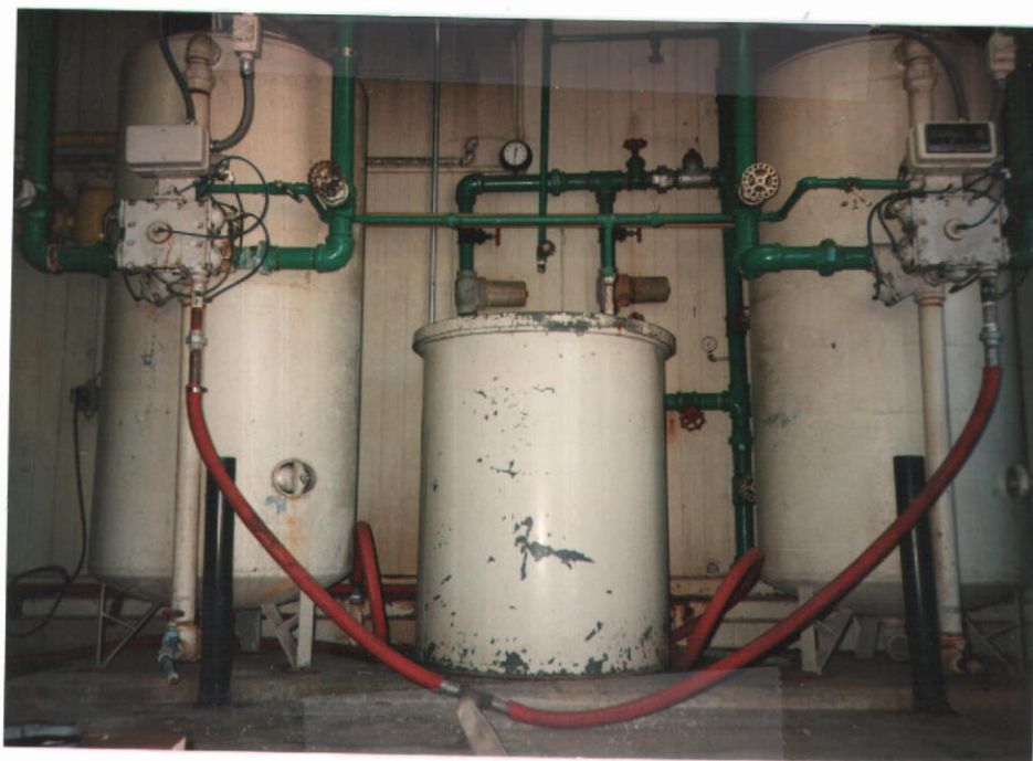
water conditioning tanks
