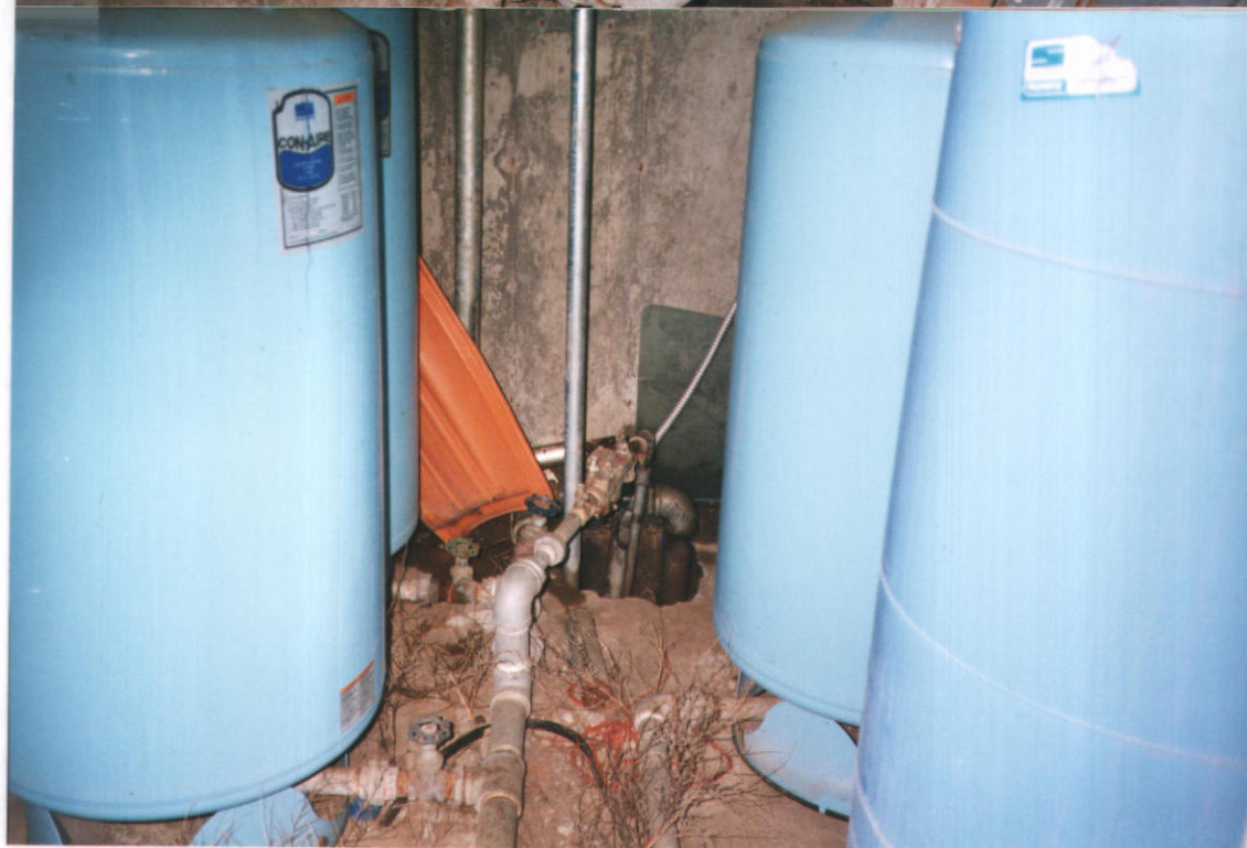
Valves & Pressure Tanks For Wells #1 & 2
