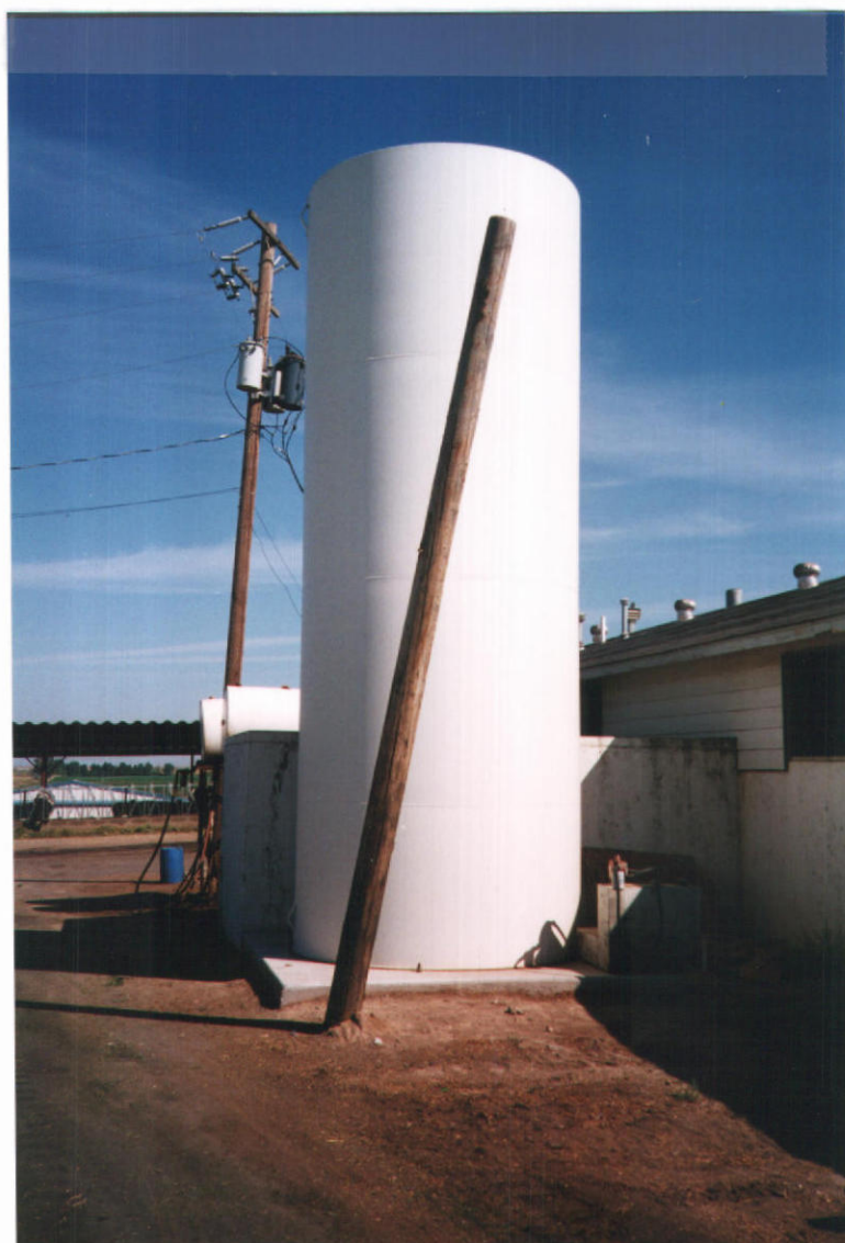
Storage Tank for Wash Pens
