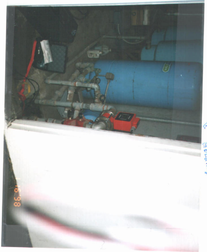
This line Feeds Balers ↓ Holding Tanks
