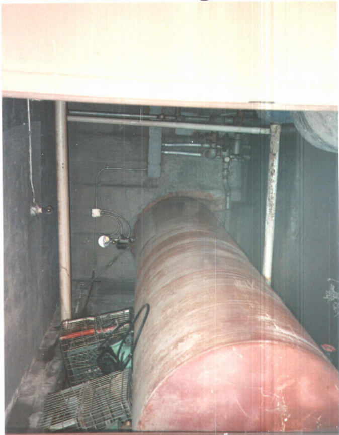
Pressure Tank w/Booster pump.
