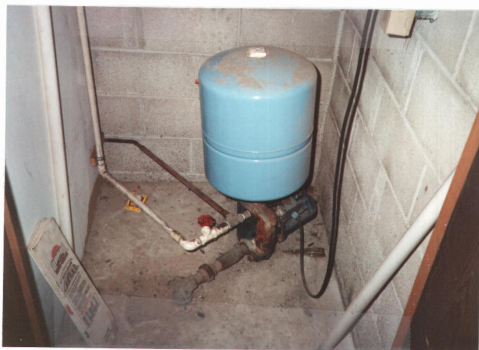
Sandpoint well & pump
