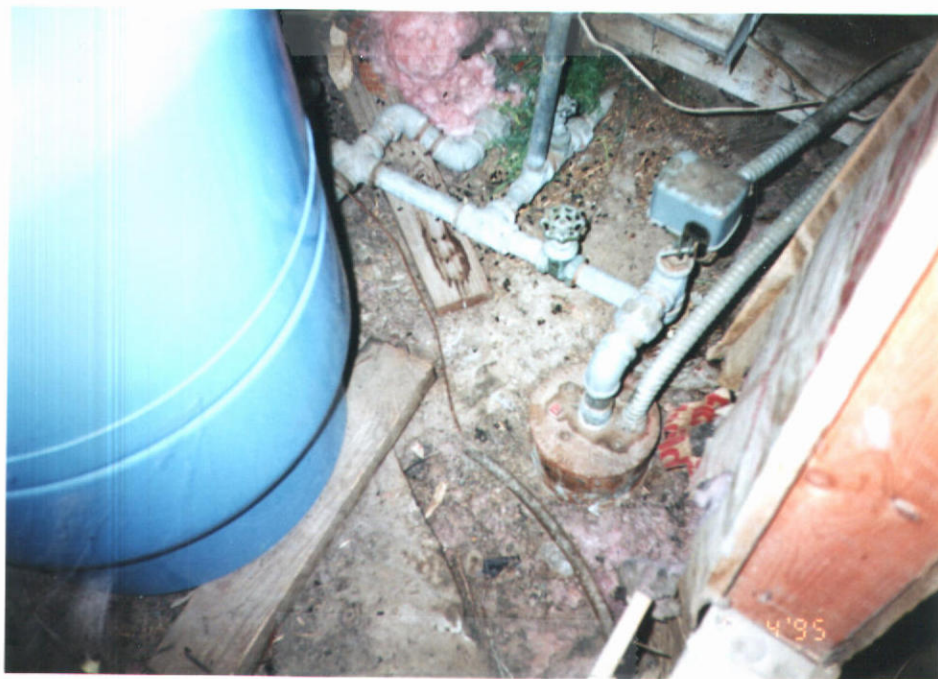
P/D (Well head & pressure tanks inside old wellhouse)
