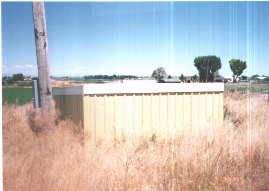
P/D #2 (Well #2; wellhead & pressure tanks inside of the metal wellhouse)
