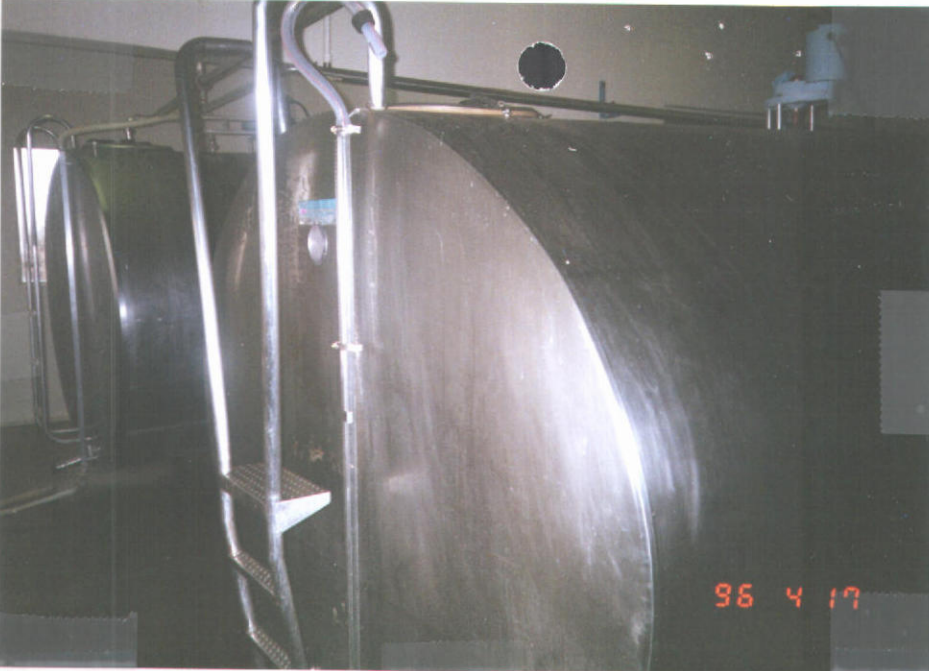
VIEW SHOWING MILK COOLING/STORAGE TANKS ON EAST END OF DAIRY BARN.
