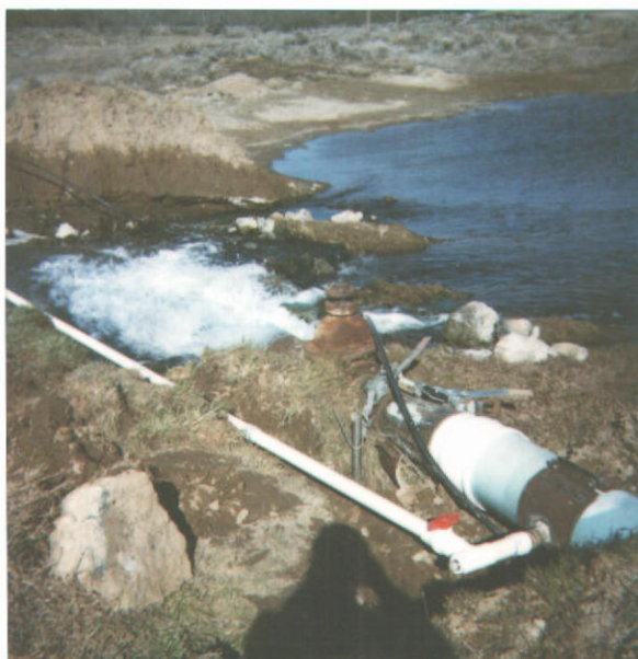
Pipeline Discharge Into Ponds, White PVC Pipe To Heat Pump
