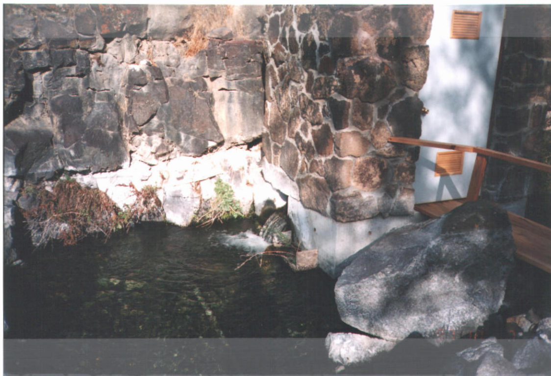
Pumphouse, Overflow From Springs
