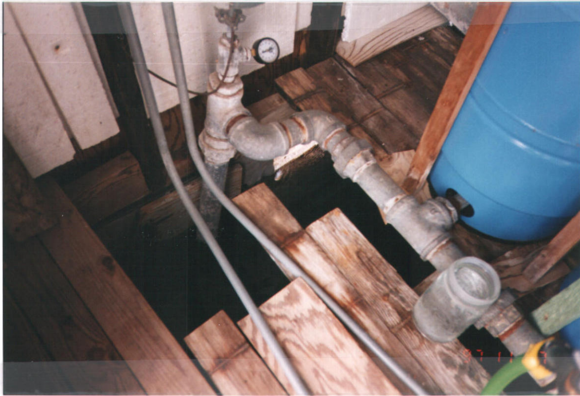
Inside of Pump house
