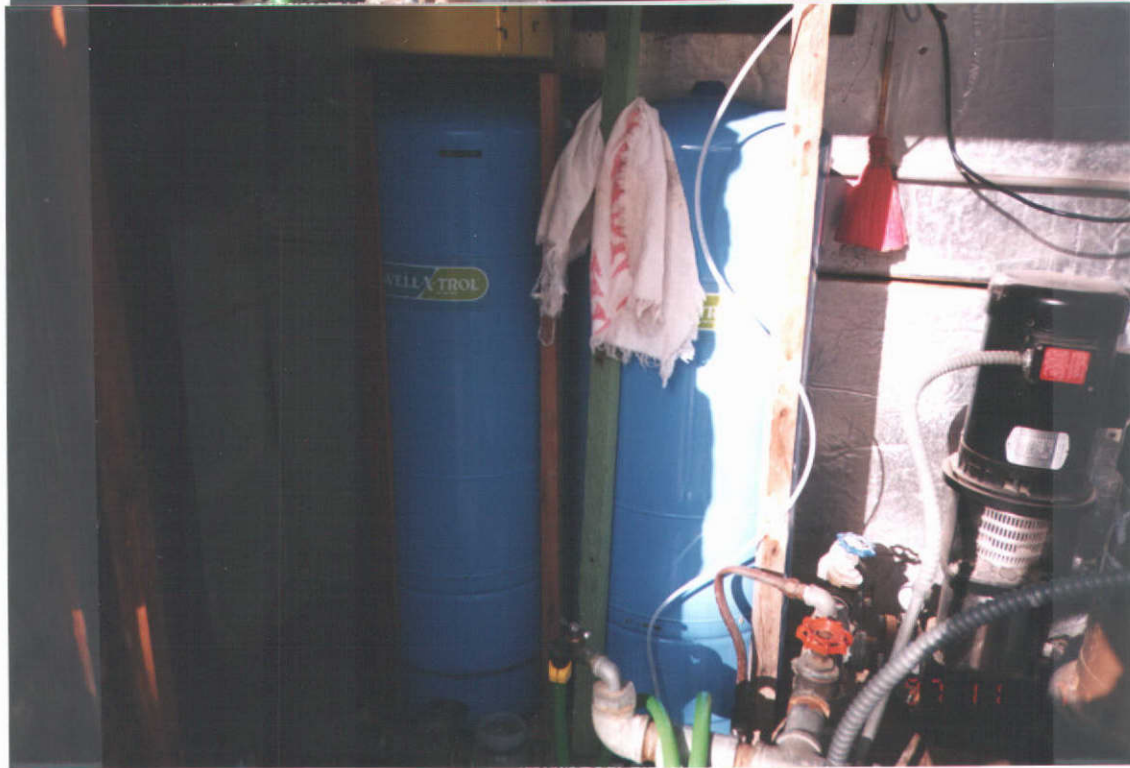
Inside View of Pumphouse
