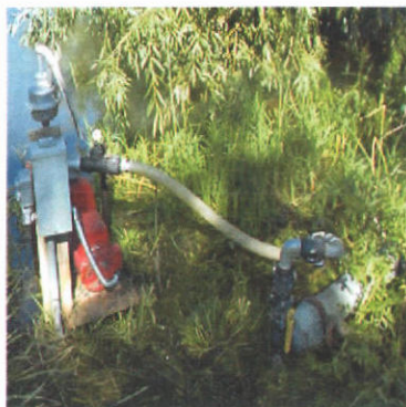
5hp pump to main line
