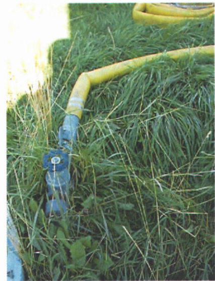
Valve from well
