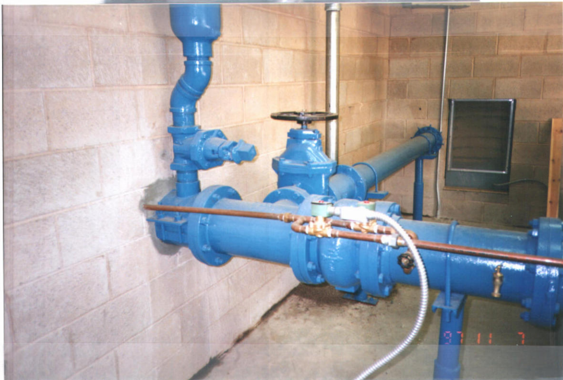
Mainline From Well Into Pump House
