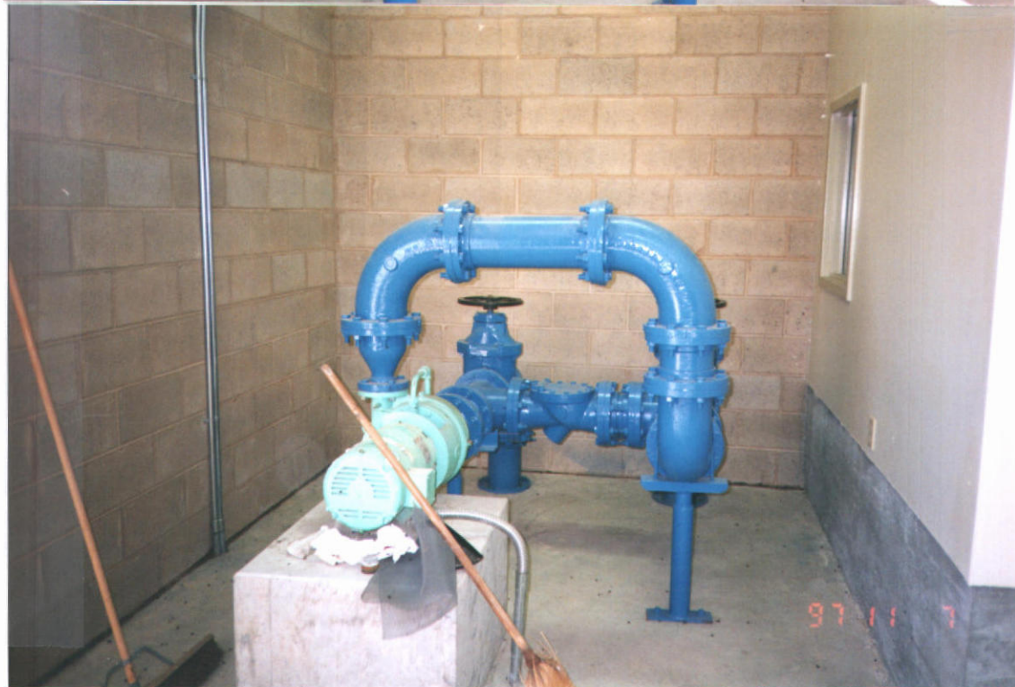
Inside of Pumphouse
