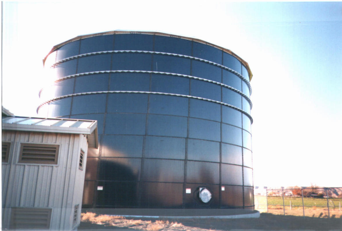
Storage Tank (Well + Pump In Metal Shed)
