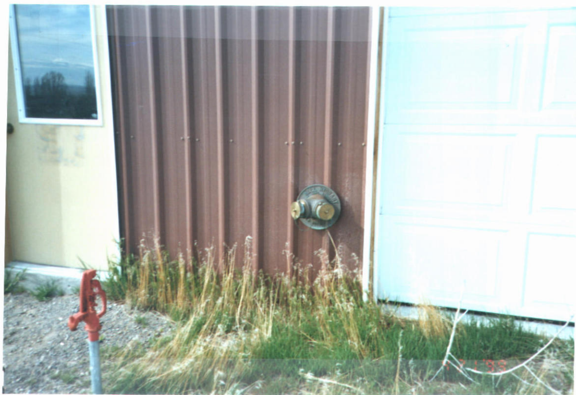
Fire Outlet Outside Pumphouse
