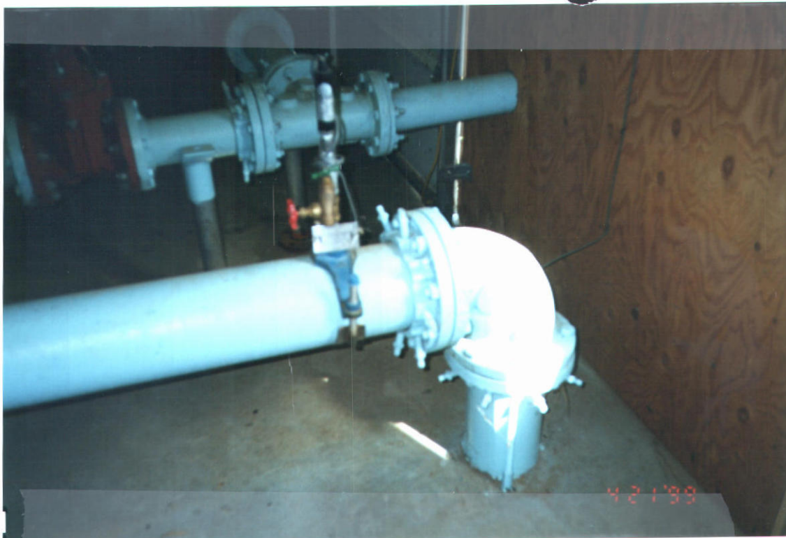
Outlet For Fire Hoses (Top Pipe)
