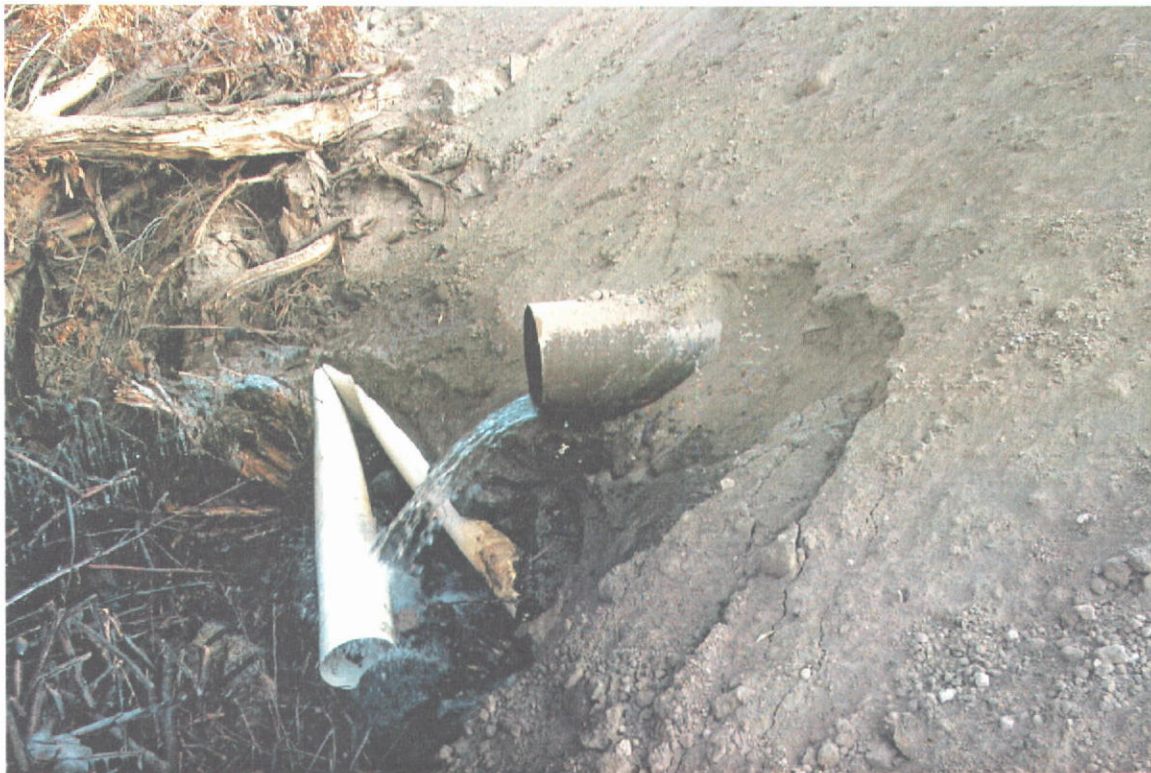
View showing the downstream end of the outlet and erosion at the toe of the "dam". Note that erosion from the outlet discharge and the steep, loose, downstream slope are causing embankment slope stability problems in this area.
