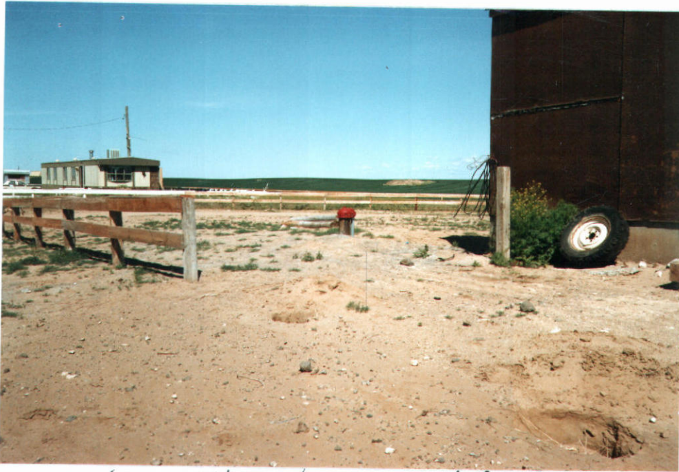
Sub. Well w/motor & Pump.
