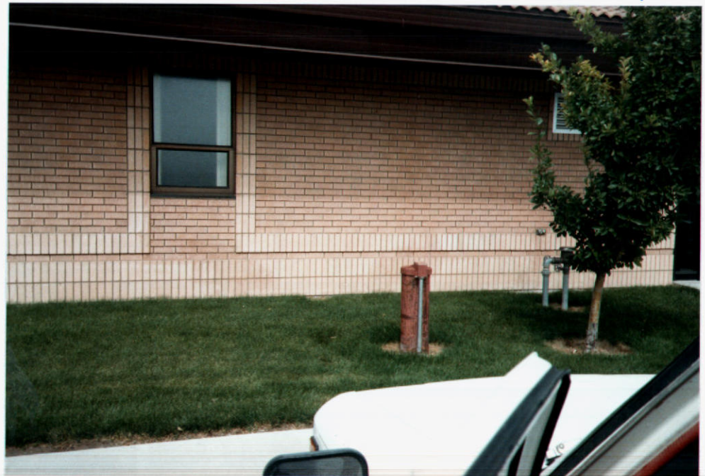
8" Dia Well w/ Submersible Motor & Pump.
