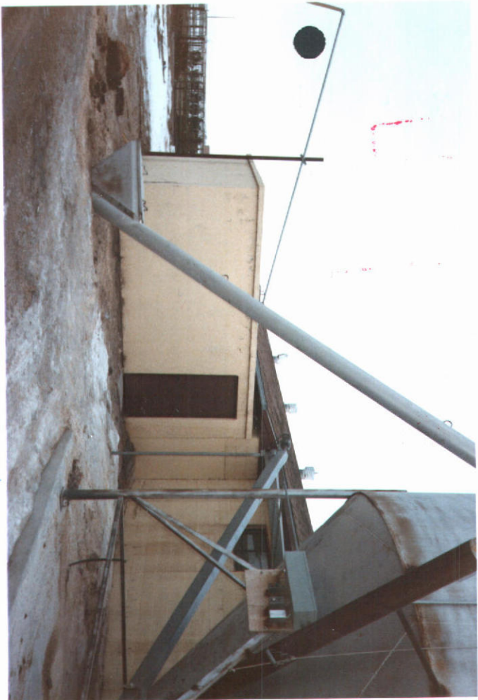
Well House w/ Storage Tank.
