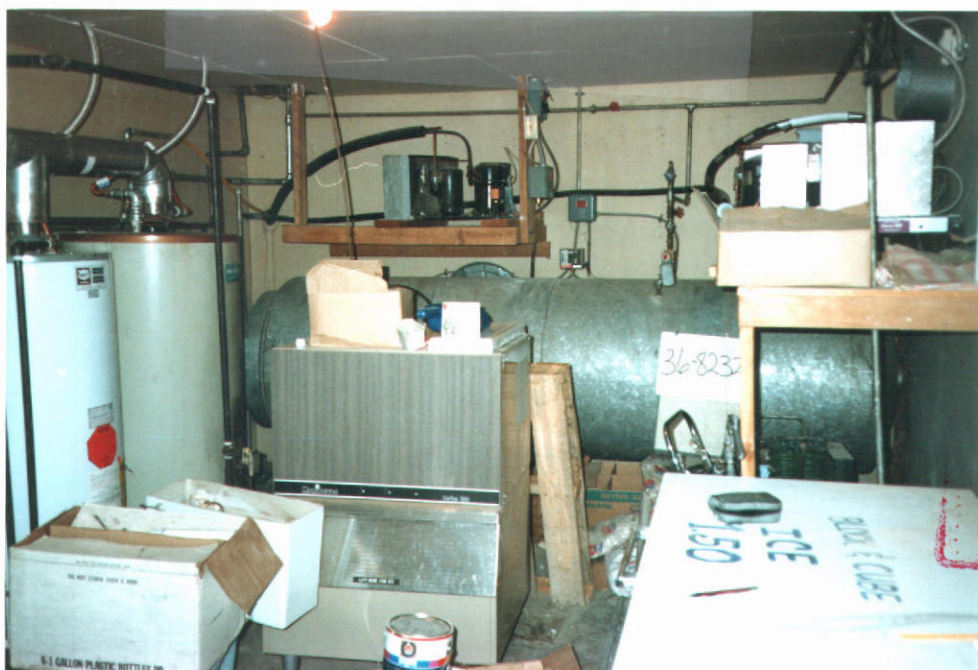
500 gal. Storage tank
