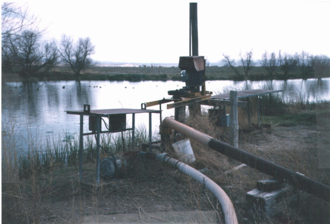
Relifts at Upper Pond 7\frac{1}{2} & 15 HP Pumps NE/4 NW/4 Sec. 12, T7S, R4E
