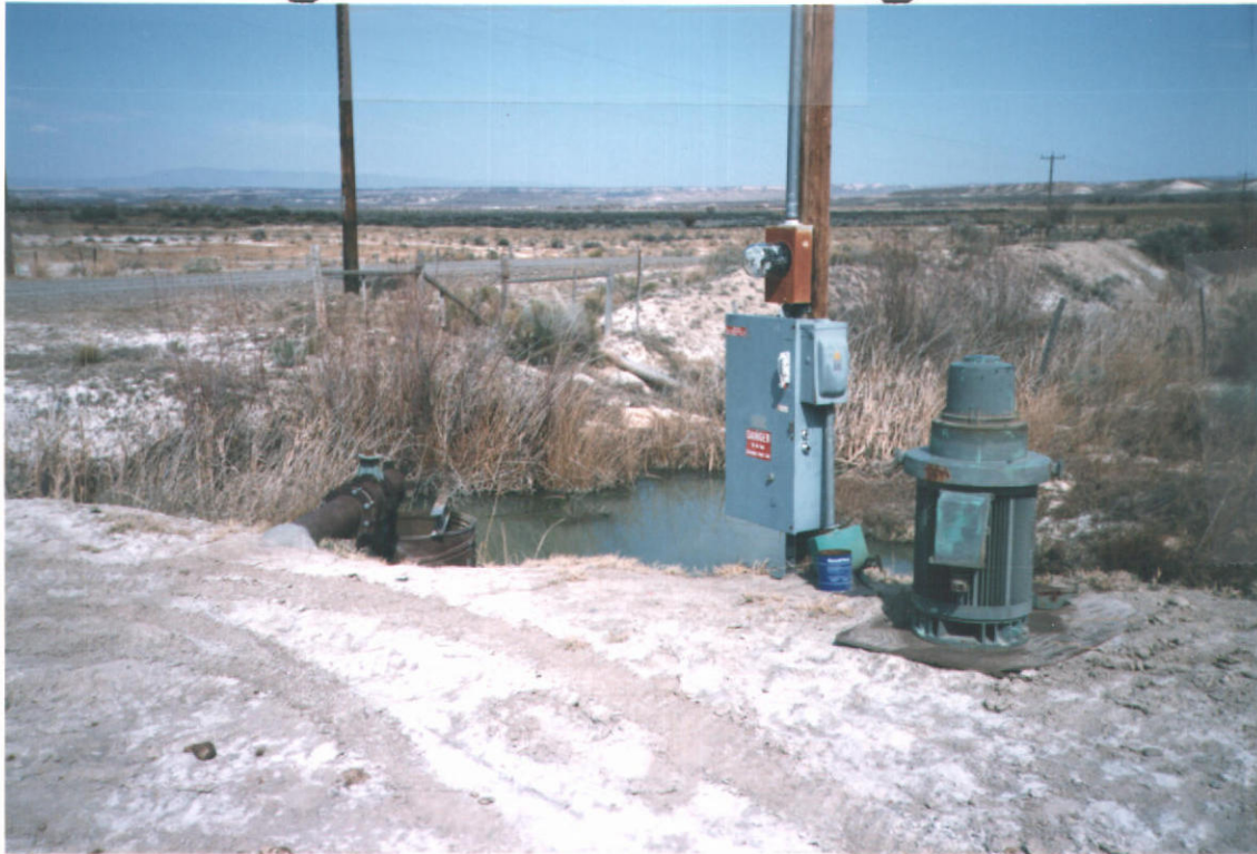
Northeast Relift Pump 60 HP
