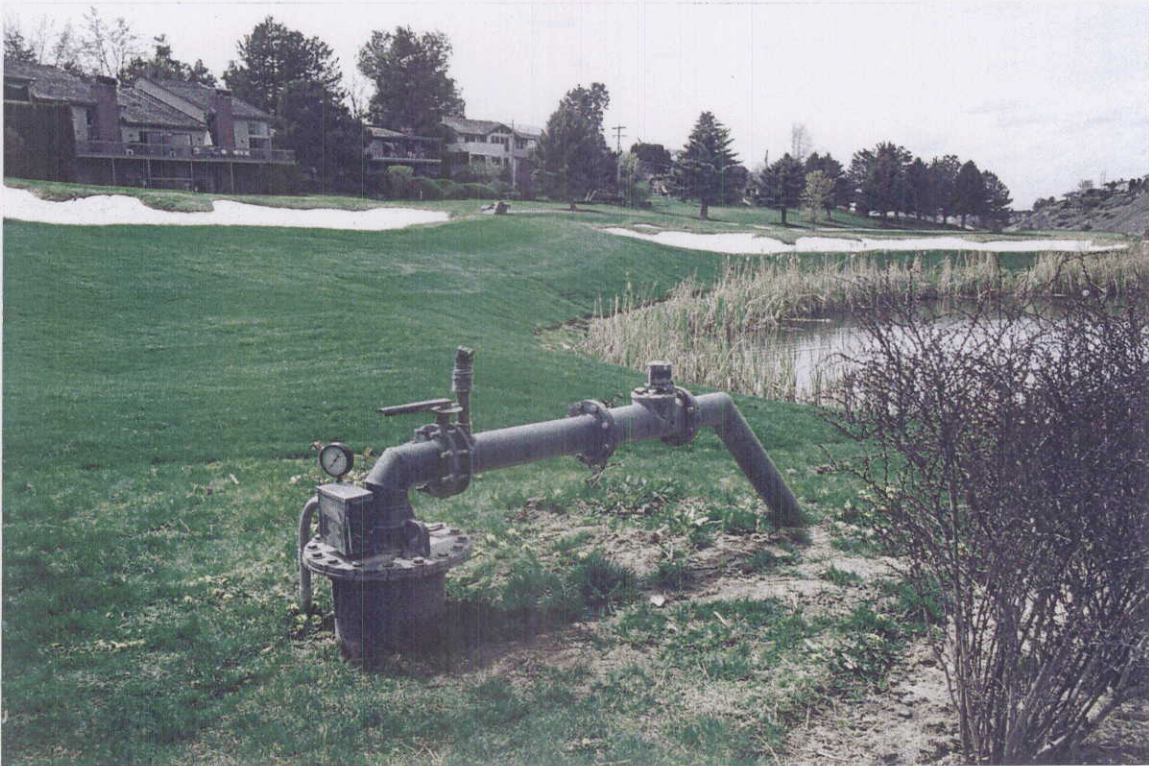
Figure 5. Photographs of the Crane Creek Country Club's Back-9 well head (2003). Upper view shows the Back-9 well's totalizing flow-meter after the pump was activated for the field examination. Lower photo is of the Back-9 well discharging directly to the Back-9 Pond at about 730 gpm. Visible are the pressure gage, control valve, and flow-meter. The well is equipped with a submersible pump and motor.
