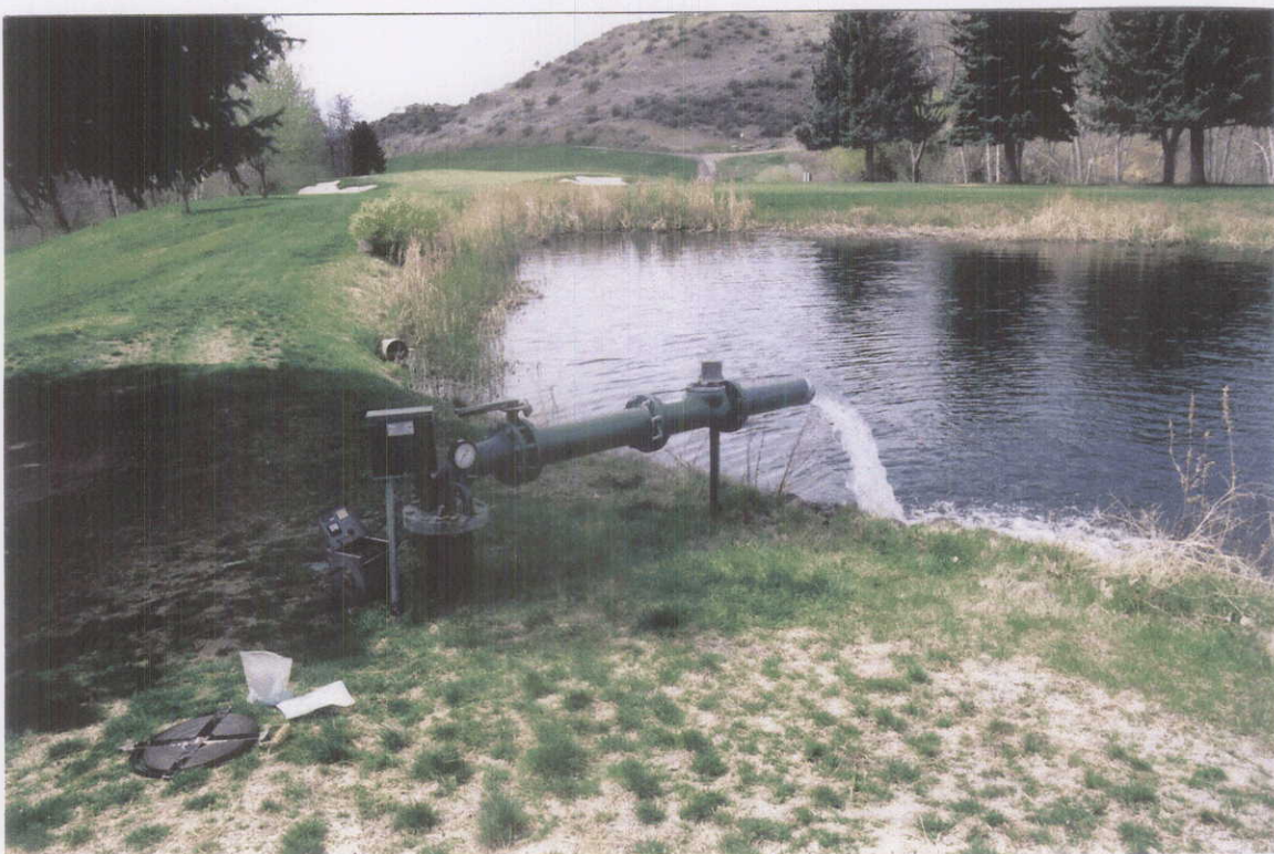
Figure 3. Photographs of the Crane Creek Country Club's Front-9 well head (2003). Upper view shows the Front-9 well's totalizing flow-meter after the pump was activated for the field examination. Lower photo is of the Front-9 well discharging directly to the Front Nine Pond at about 550 gpm. Visible are the pressure gage, control valve, and flow-meter. The well is equipped with a submersible pump and motor.
