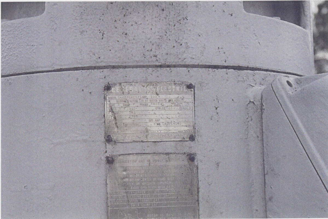
Figure 7. Photographs of the CCCC Club House Well's well head. Upper view shows the G.E. drive motor for the line-shaft turbine pump and the 6-inch diameter discharge piping which houses the totalizing flow-meter. Lower picture shows the motor specification plate for the 100 HP drive motor.
