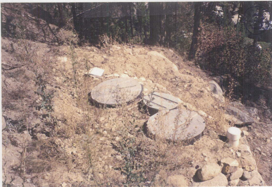
③ Storage tanks for Cross + Hartung - for compressed water. gravity flow from here back down to cabins.
