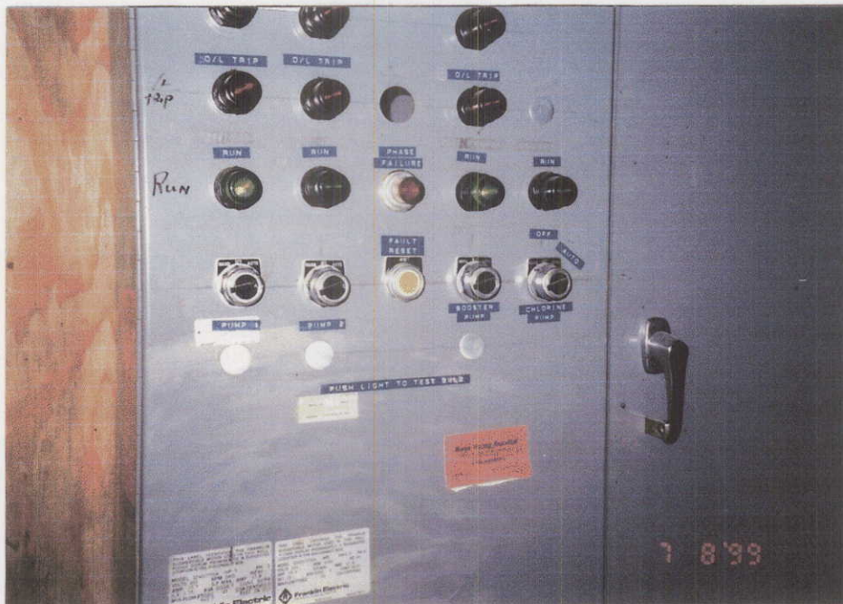
Control Panel on North Wall of Well House
