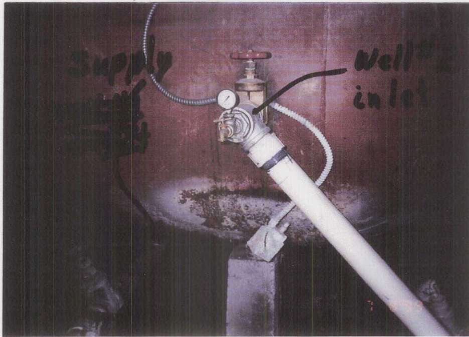
Inlet to 2000 gal Storage tank
