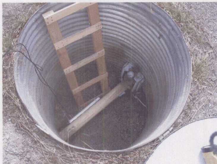
Meter Vault - Meter = 4" McCrometer Serial #97-8151-4
