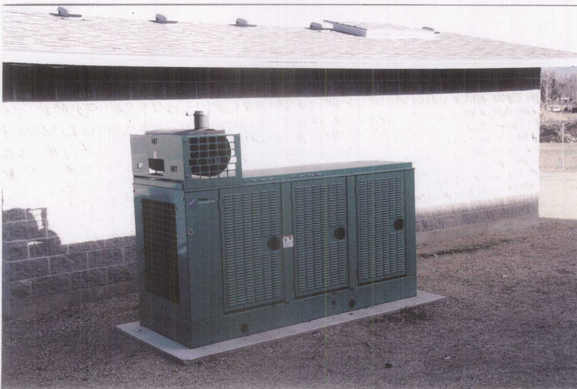
Figure 8. February 11, 2005 photographs of the Toshiba adjustable speed drive installed on the City of Meridian's #21 municipal water supply well (upper) and the Cummins 150 KW, natural gas powered electrical power generator for use in emergency power outages (lower).
