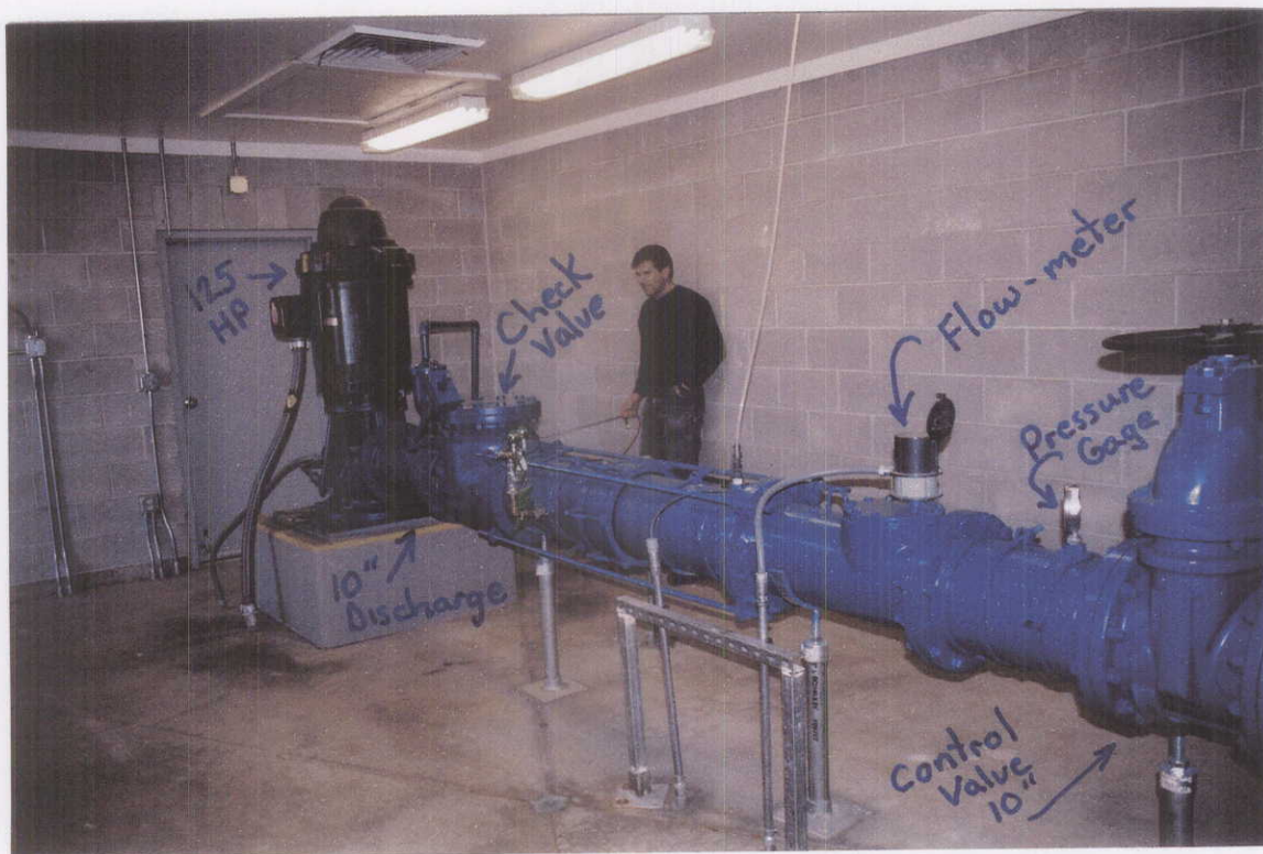
Figure 3. Photographs of the well head plumbing inside of the Meridian Well #21 pump house showing the configuration and specifications of the installed totalizing flow-meter.
