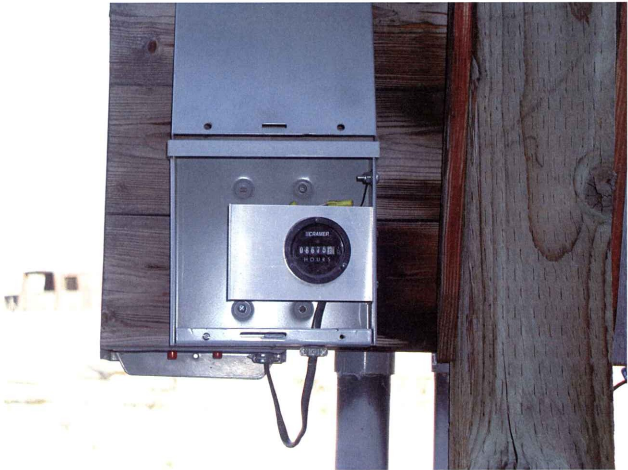
Elapsed Time Meter (Units in hours) for Williams Lake Recreational Water & Sewer District for water rights 75-7589 & 75-7590.
