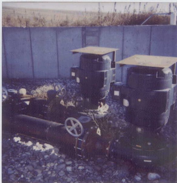
Re-lift Pumps From Pond to Sprinklers
