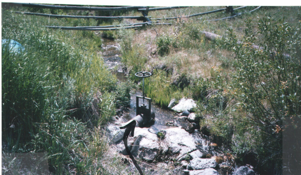
OUTLET TO CREEK
