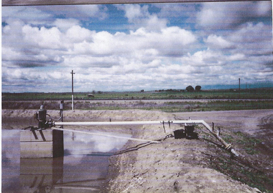
Discharge pump, measuring point looking W.
