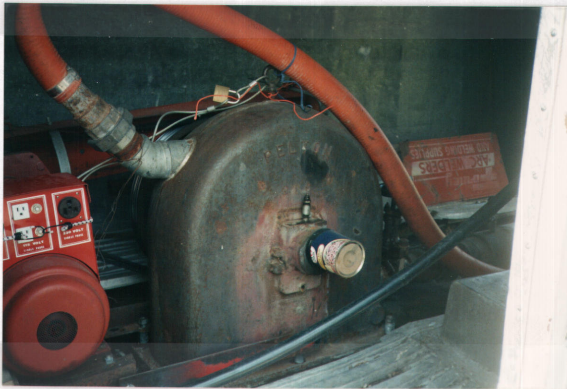
Fig. 4 - Second view of Pelton Wheel from door of powerhouse.
