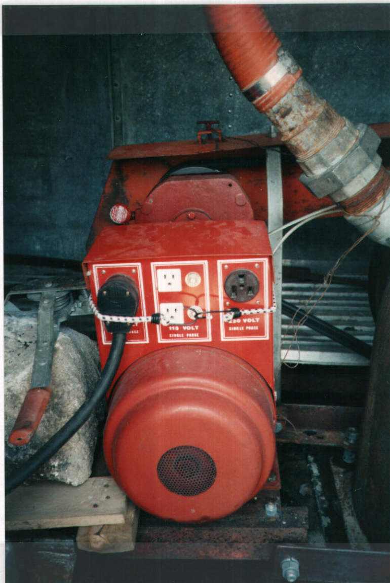
Fig. 6 - Close-up of generator operated by Pelton Wheel.
