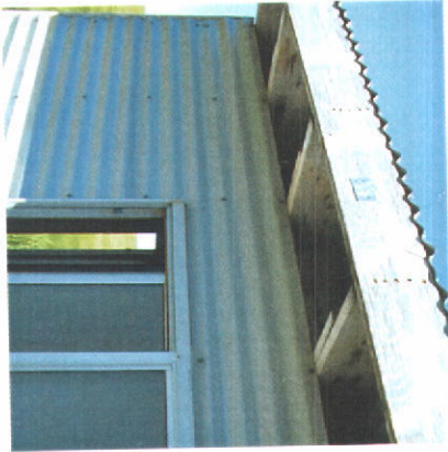
GPS Tag #A0007986 on outside of pump house
