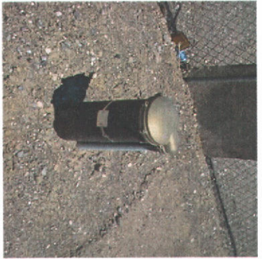
Heating Well A0007984
