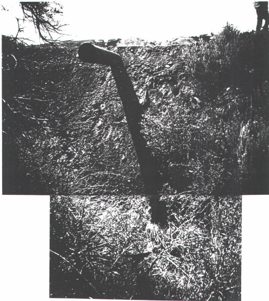
LEFT: View of the downstream slope of the embankment from the creek channel below. The maximum vertical distance between the downstream toe of the embankment and the steel pipe is about nine feet. Note some seepage water (indicated by arrow) flowing in the creek channel below the embankment.
