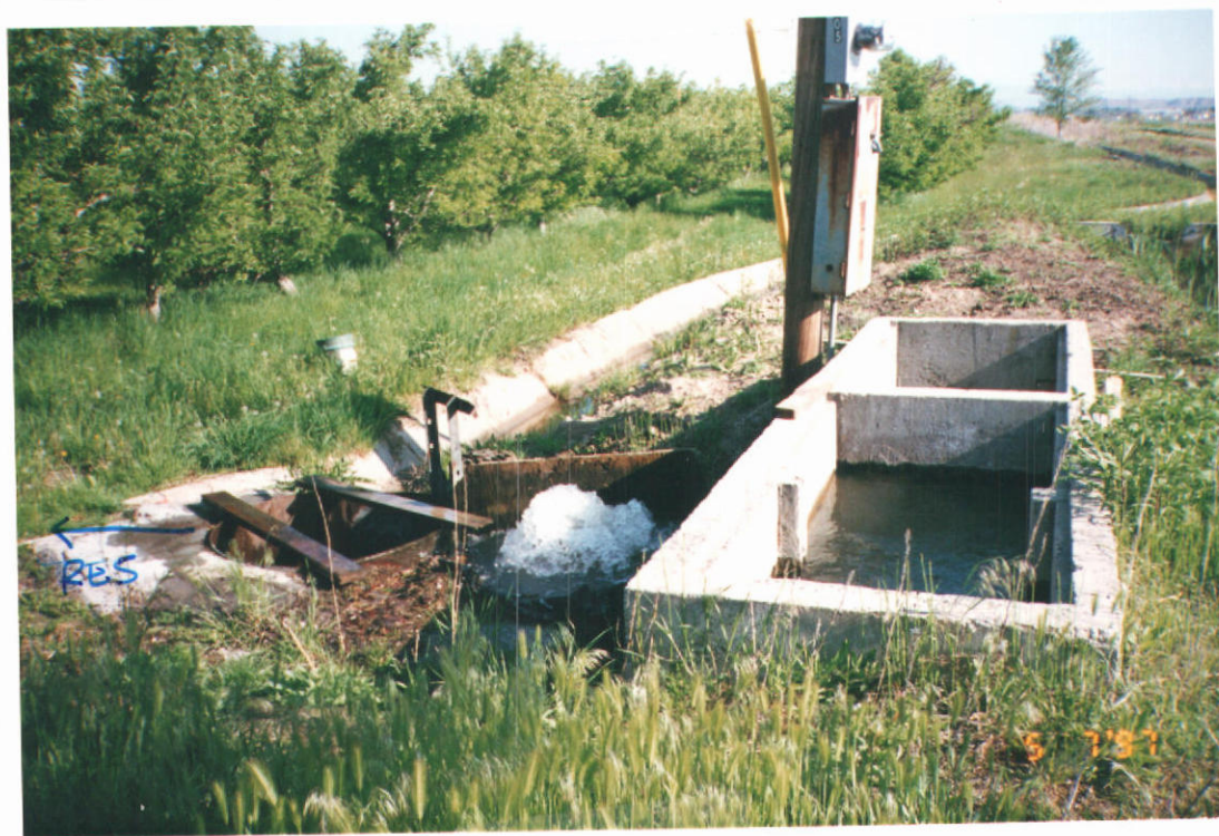
Black Canyon pick-up station in SWNE S10. (P/O for 65-5893?) overflows exit west to reservoir
