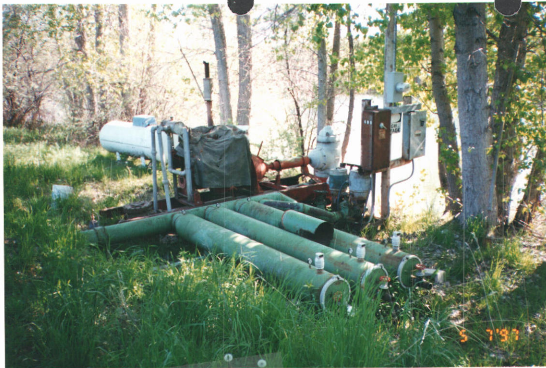
Lift station for irrigation from storage. Large pump used for frost control. Also a P/D for 65-7609 (small pumps only)
