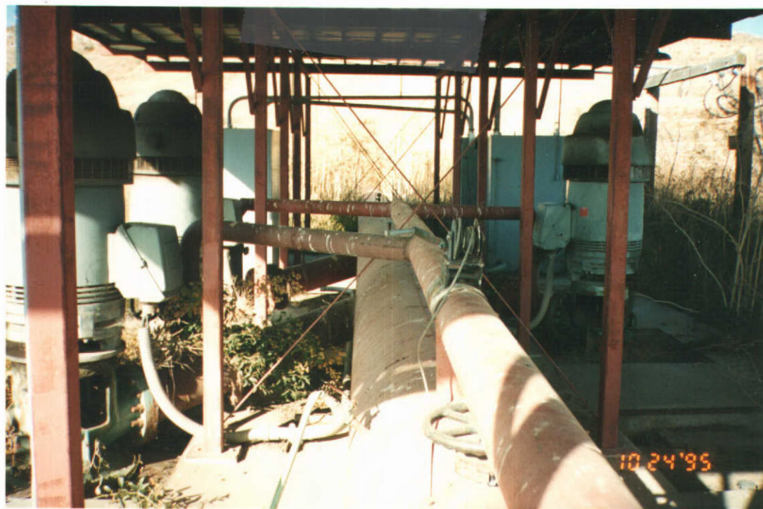
Pump Station three 300 HP Rayne Pumps
