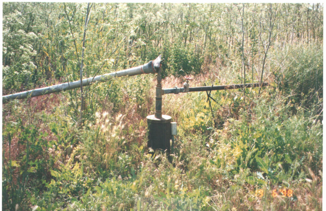
one of three wells in NESE, sec 17 feeding intern
