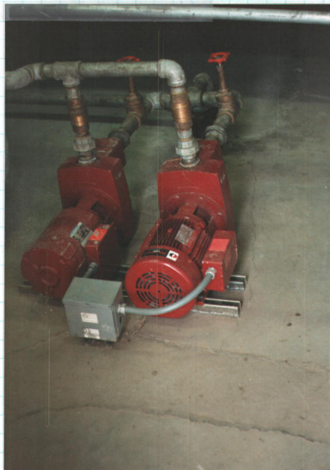
DUPLEX BOOSTER PUMPS
