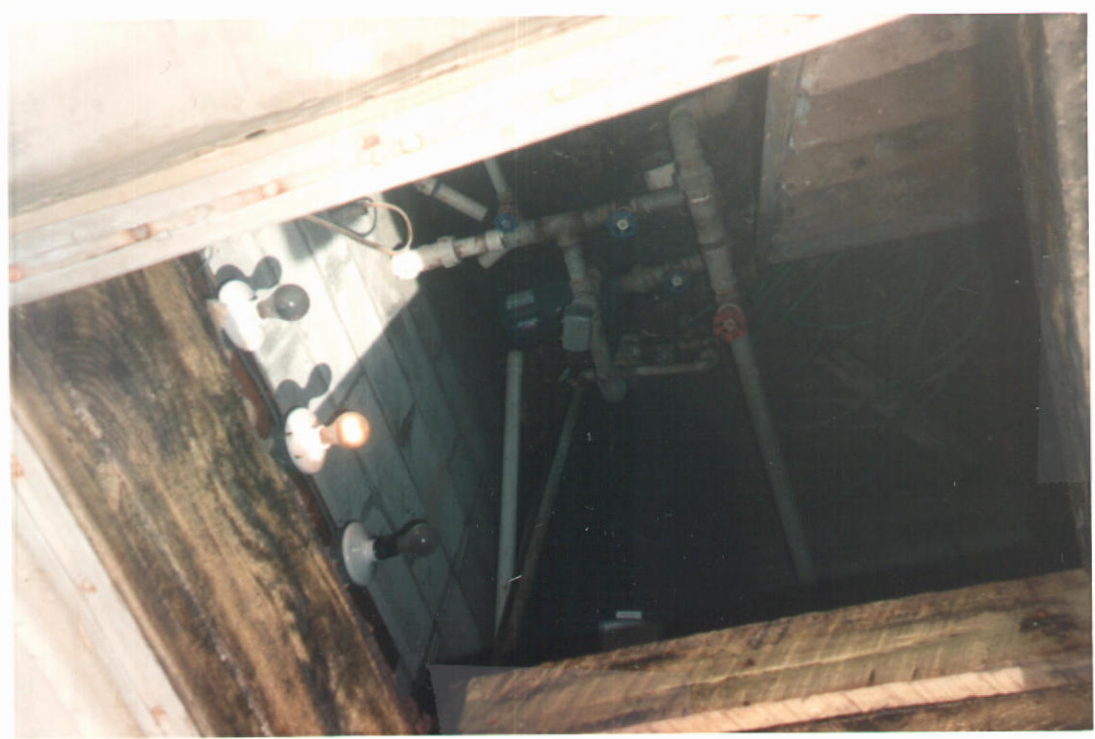
Inside Motor and piping housing. Pressure tank connected to line to house only.
