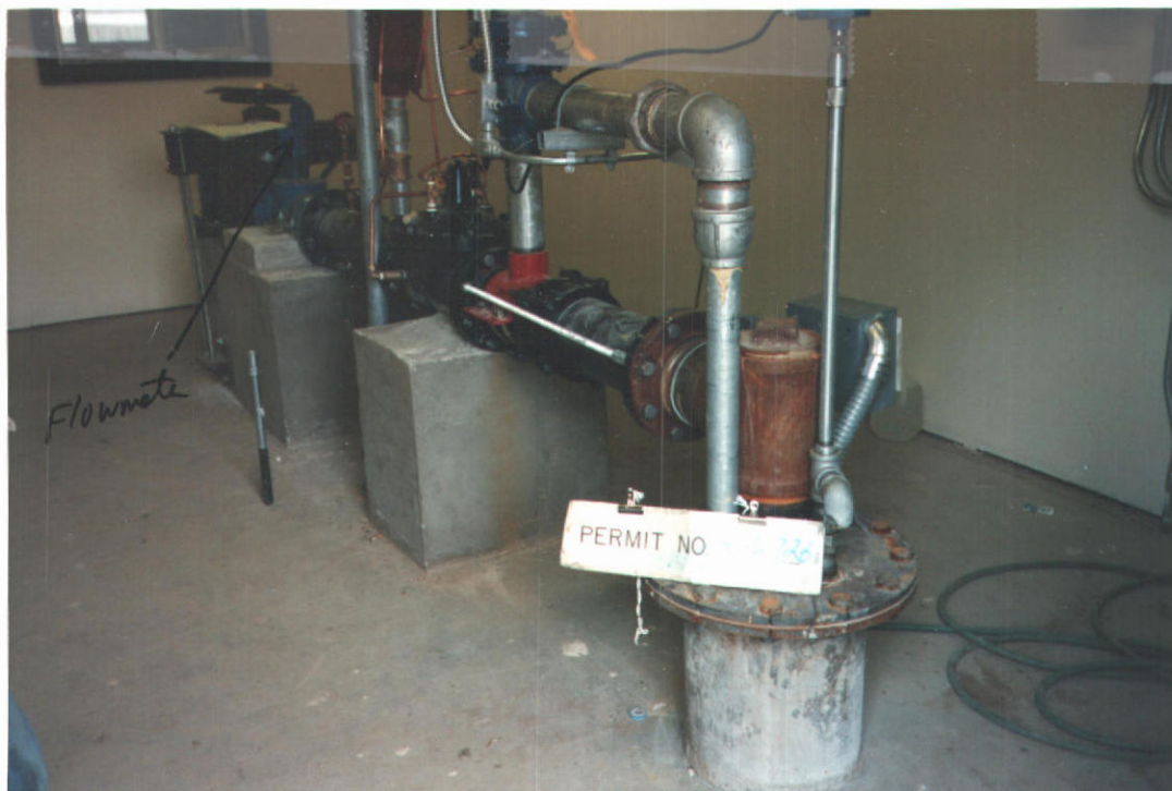
PHOTO THREE- Another view in pump house.
