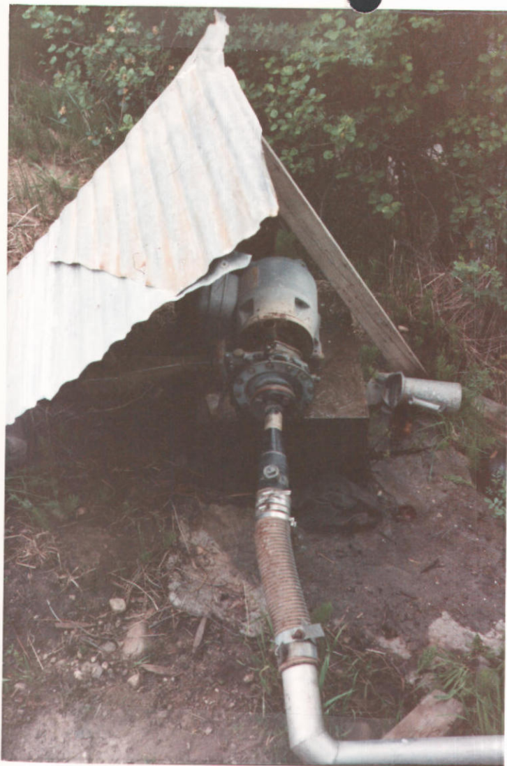
3HP Westinghouse Life Line Pump ser # 13-36V52 style 1365269
